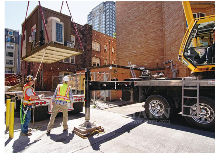
The number of VRFs installed in the United States is increasing
